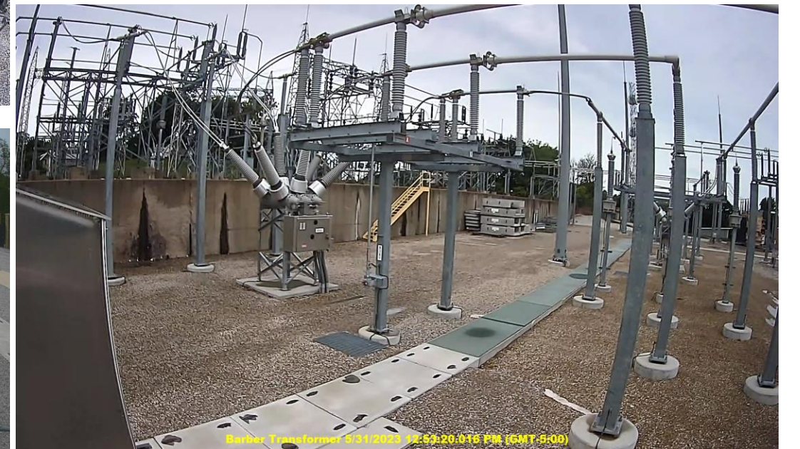
Barbet Transformer 5/31/2023 12:53:20.016 PM (GMT-5:00)
