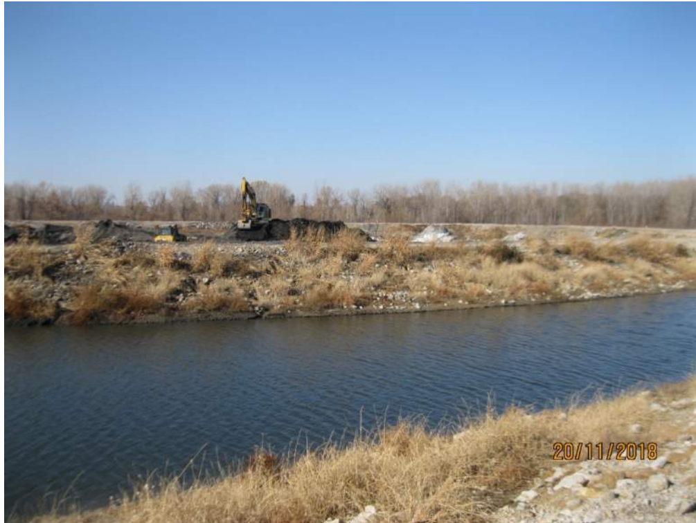
Figure 4 – Interior Slope of Clear Water Pond without Rip Rap.
