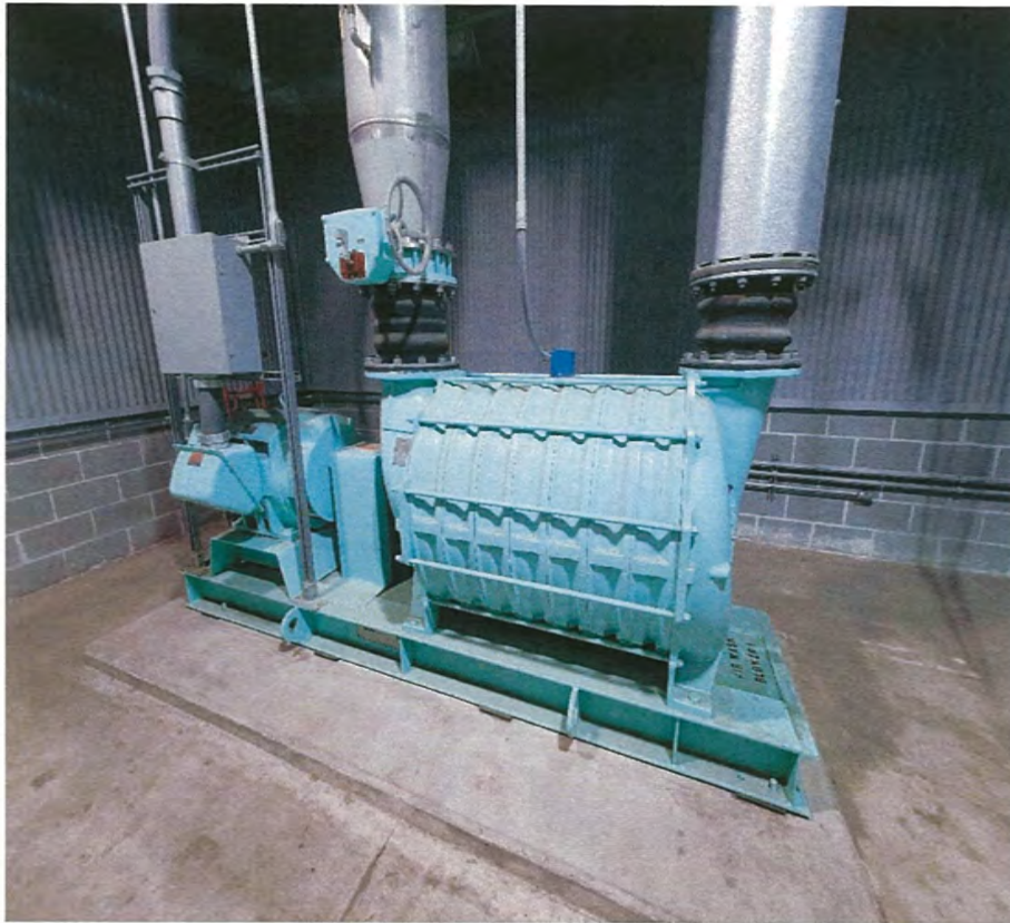
Old blower unit before rebuild
