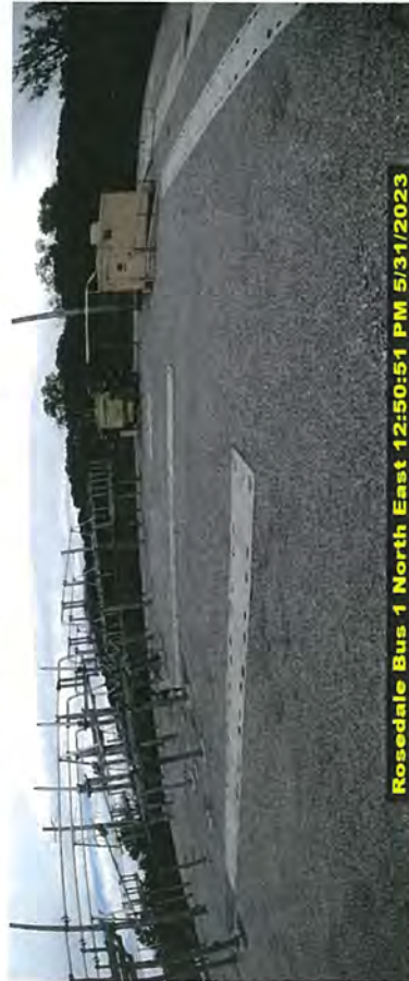
Transformer Enclosure 5/31/2023 12:50:51 PM (GMT-5:00)
